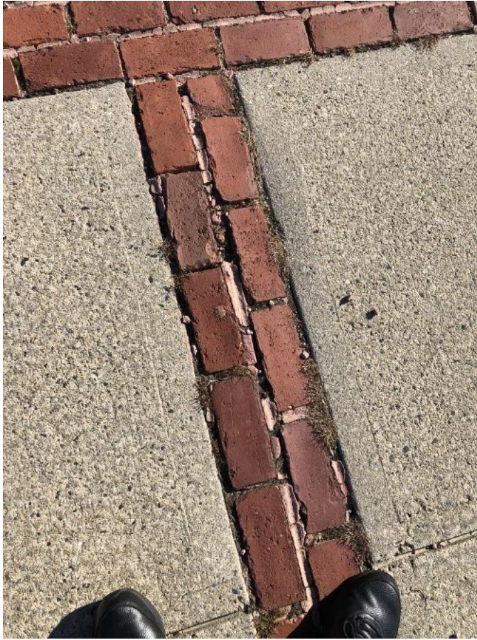
A closer view of the bricks lining a cement walkway to Corpus Christi Parish. The edges of the bricks have been broken in some areas.
