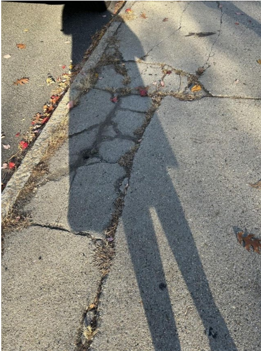
A cracked, uneven sidewalk in the path of travel to Saint Paul's Parish in Holyoke.
