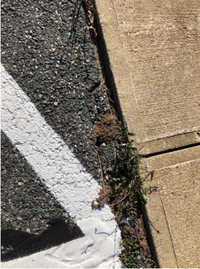
Gap between sidewalk and pavement at the Mashpee Senior Center.
