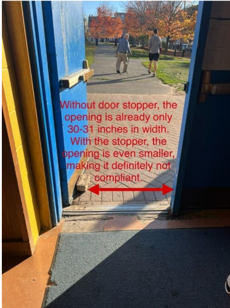
The doorway leading into East Boston High School. The door is held open with a block which partially blocks the doorway. The surveyor noted: Without a door stopper, the opening is already only 30-31 inches in width. With the stopper, the opening is even smaller, making it definitely not compliant.
