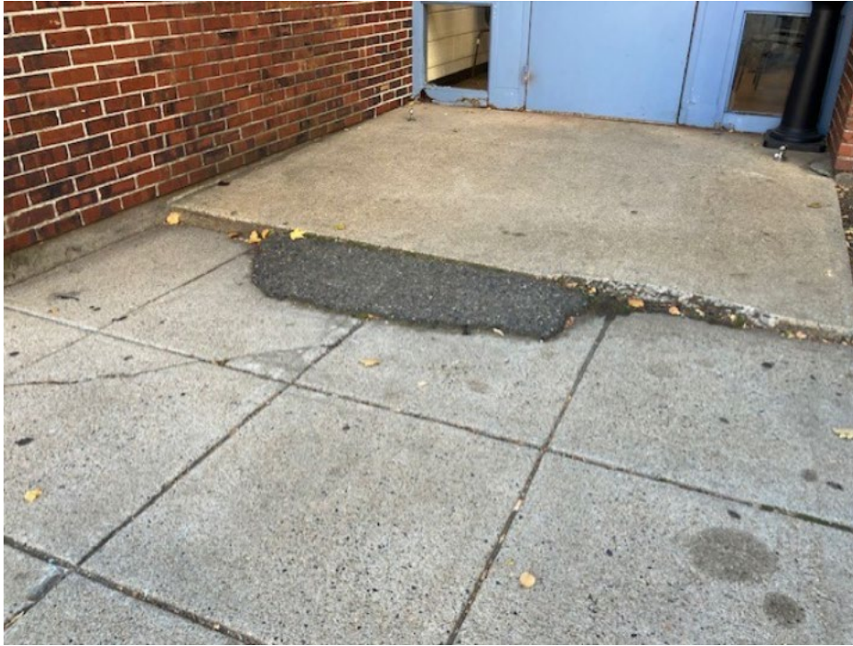
Concrete area outside of the entrance to the Salvation Army polling site. The space between the landing and the walkway has been patched unevenly with pavement, lacking a compliant ramp.
