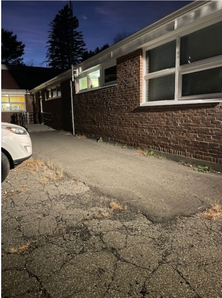
The path of travel at the back of Washington Town Hall leading to the accessible entrance. The area has broken and patched pavement.
