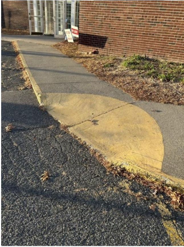
Sidewalk leading to the Sturbridge Post Hotel with a makeshift curb cut. The threshold between the curb cut and parking lot interrupts the path of travel.
