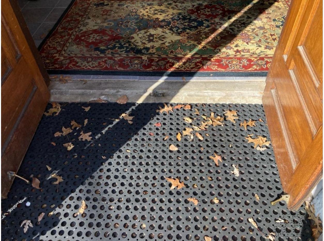
Saint Mary's entry doorway from the exterior area in front of the doors. A black rubber mat is placed in front of the doors and threshold which measures over ½ inch above the ground.
