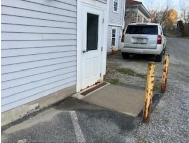
Side view of the exterior entrance to the Tyringham Town Hall. The threshold to enter is over one inch above the ground.
