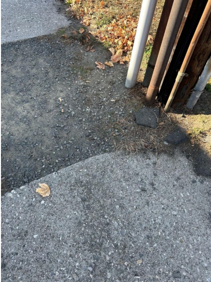
Patch of sidewalk in Holyoke where the pavement suddenly ends is filled with gravel and dirt, creating an uneven surface.
