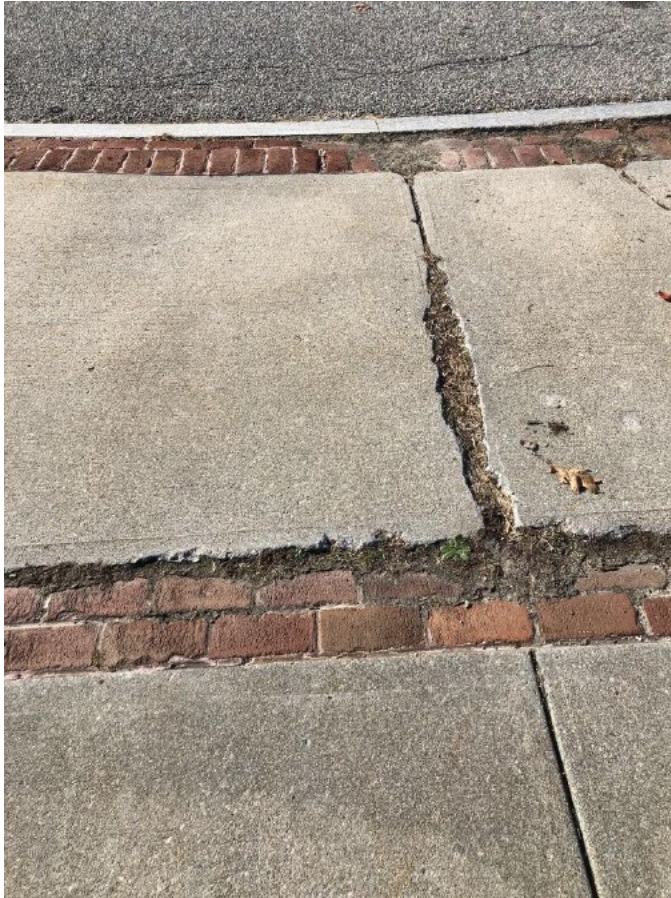
The path of travel at Corpus Christi Parish Hall. There is a relatively flat curb next to the paved parking lot. Bricks line the cement sidewalk. There are cracks deeper than \frac{1}{2} inch in the cement sidewalk and bricks.
