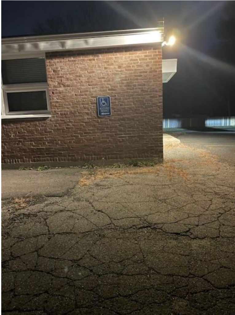
The back of Washington Town Hall during the evening. The area around the building has broken and patched pavement. A sign posted on the building directs voters to the accessible entrance.
