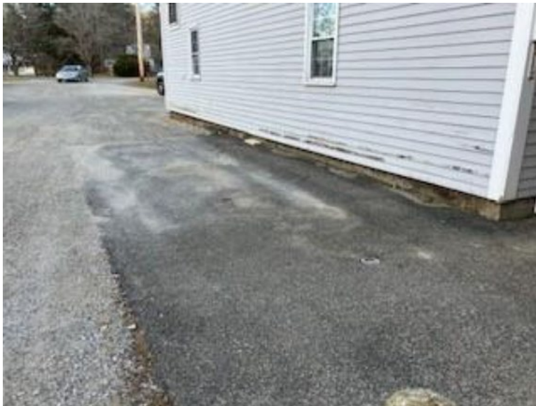
Side of the Tyringham Town Hall and part of the parking lot. The parking lot is partially paved on the perimeter of the building, while the rest of the parking lot is gravel. There are some uneven areas in the parking lot.
