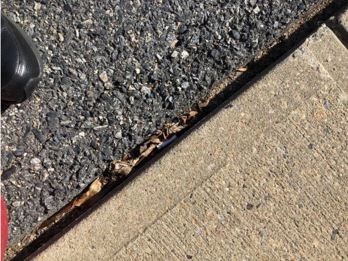
Gap between sidewalk and pavement at the Mashpee Senior Center.
