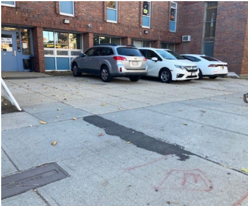
Parking lot behind the Salvation Army in Cambridge. There are several cars parked along the building and some patched pavement. No HP signs or striping are visible.
