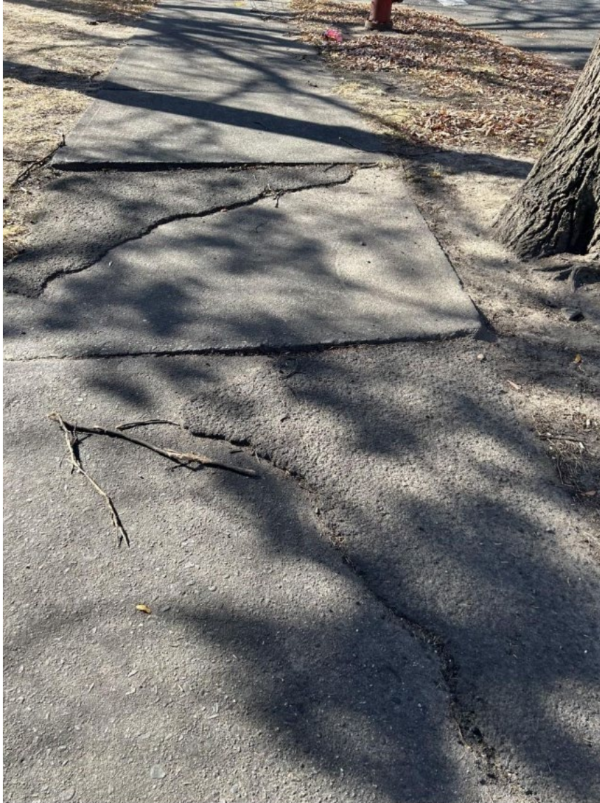
The sidewalk leading to Saint Paul's Parish. There are several cracks and uneven areas in the sidewalk, including areas where the sidewalk is lifting or where patches in the pavement create an uneven surface.
