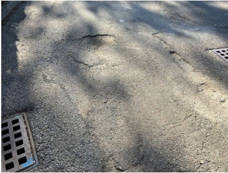
Parking lot leading to the Arlington Town Hall. Cracks and holes in the pavement are greater than ½ inch deep.
