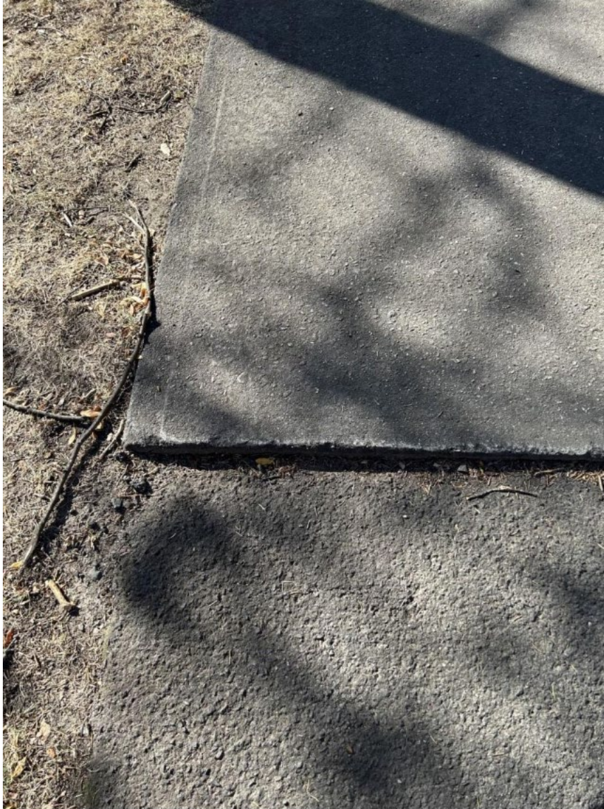
A cement slab of sidewalk in the path of travel to Saint Paul's Parish. The sidewalk is partially lifting, creating a change in level of over ½ inch.
