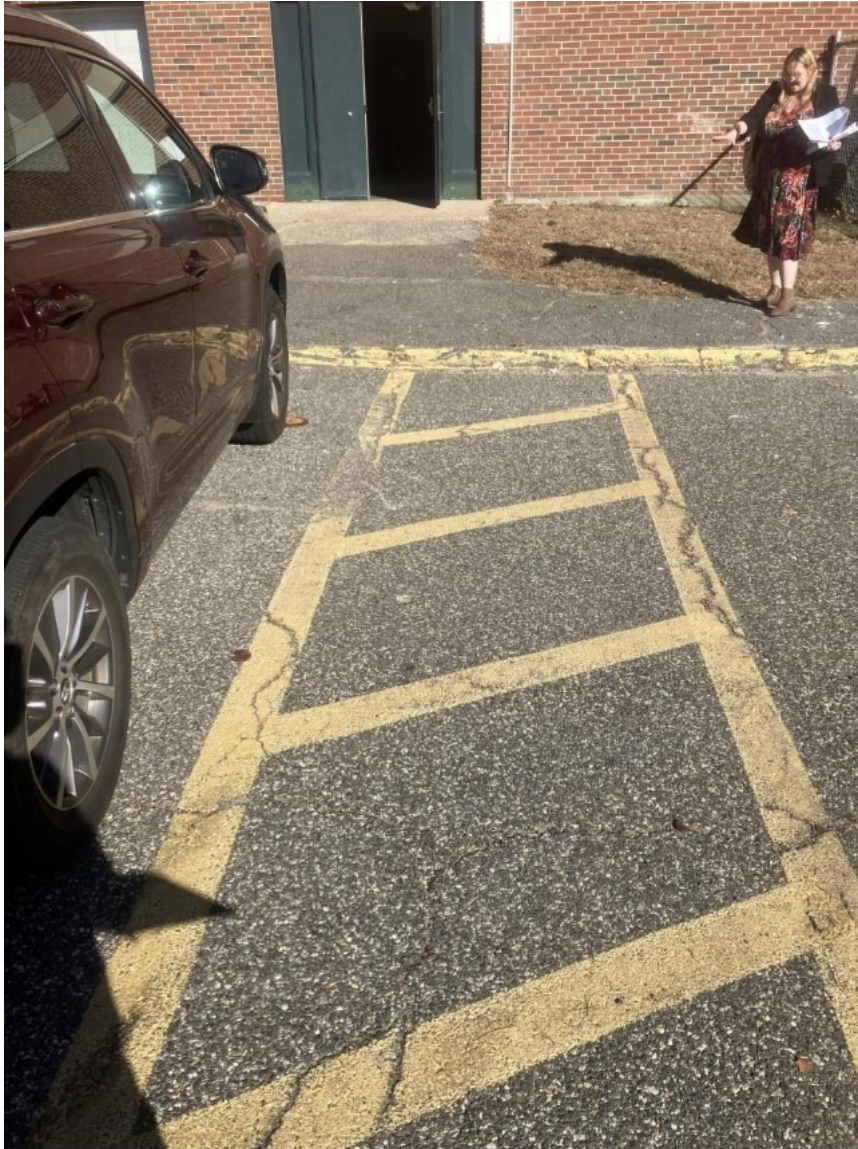
An accessible parking space and yellow striped access aisle leading to a curb in front of the polling place entrance. There is a yellow painted curb directly in front of the accessible parking space and no curb cut.
