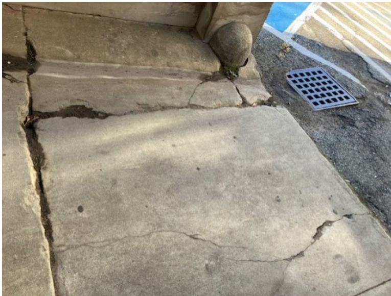
Cement walkway leading to Arlington Town Hall. The cement is very cracked and broken in several areas, leading to abrupt changes in level greater than ½ inch.
