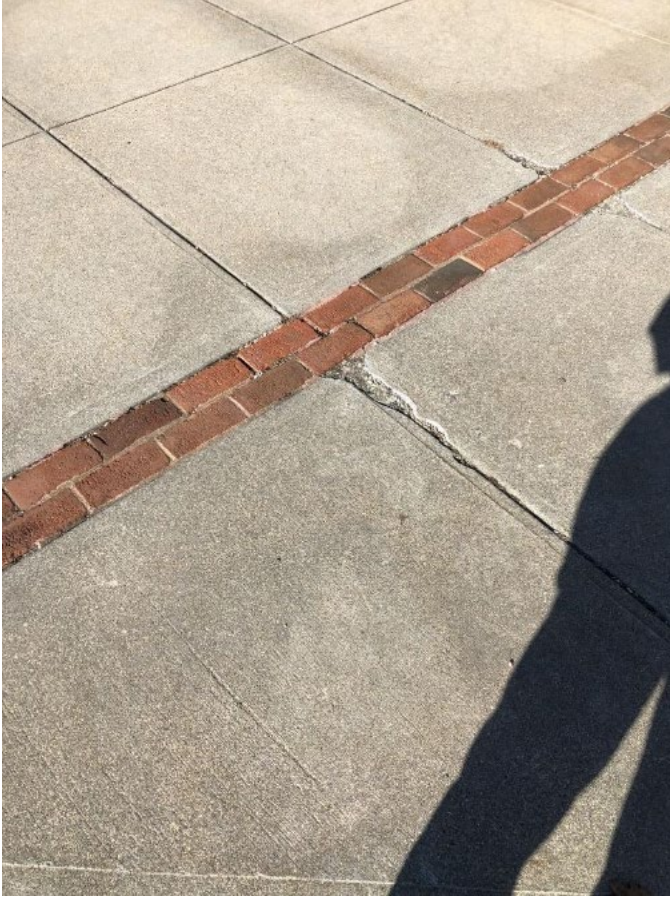
The path of travel to the Corpus Christi Parish Hall. There is a crack in the cement walkway.
