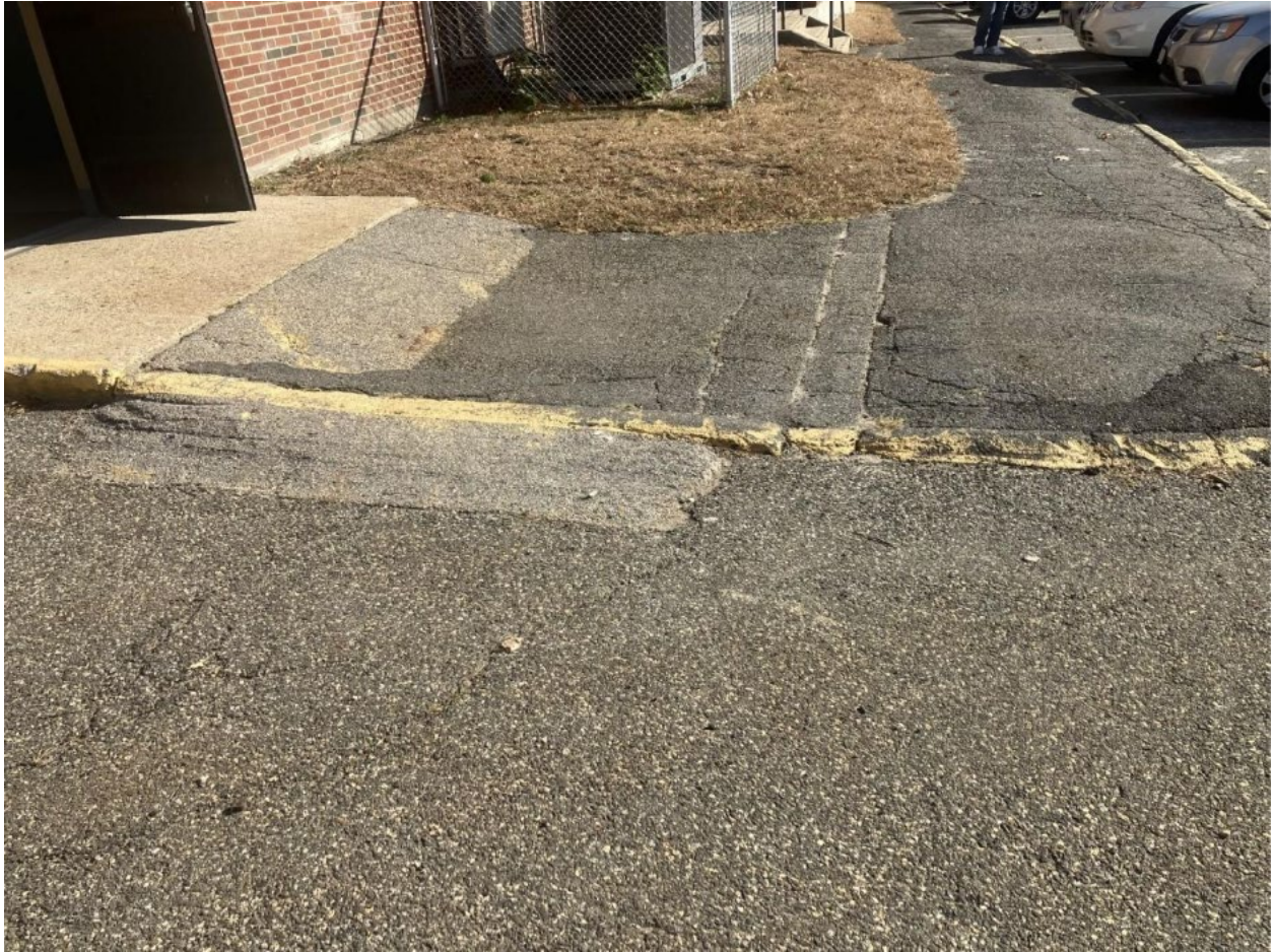
A closer view of the pavement in the path of travel to the polling place entrance. The pavement is uneven and cracked in multiple places and lacks compliant curb cuts.
