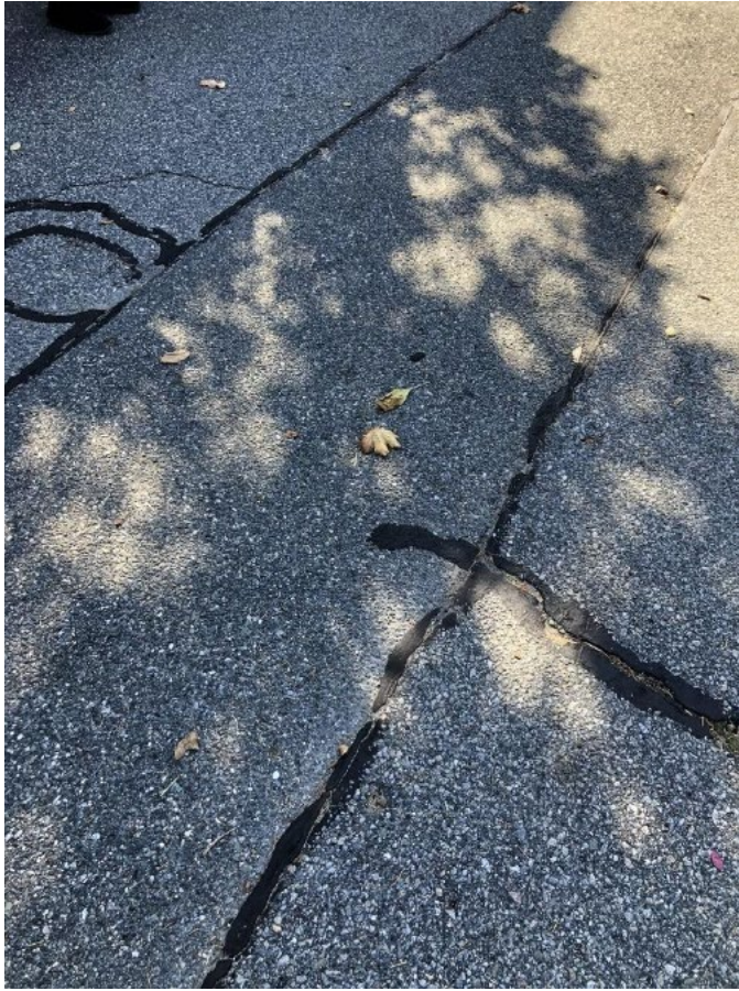
Pavement near the Mashpee Town Hall. There appears to be a slight incline. The pavement has some cracks and patching.
