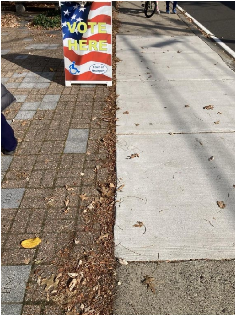
A sidewalk lining the street next to Saint Mary's in Rockport. There is an area of brick next to the cement sidewalk with a difference in level greater than half an inch.
