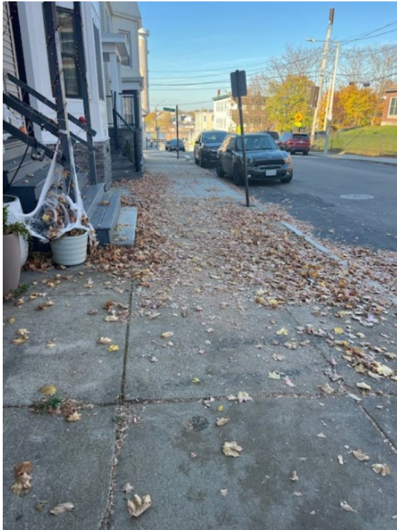
Uneven sidewalk in the path of travel to East Boston High School.
