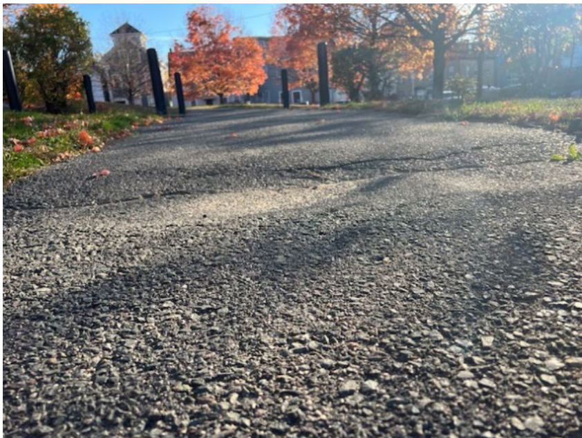
A paved walkway leading to the East Boston High School polling site. There are some cracks and changes in level in the pavement.
