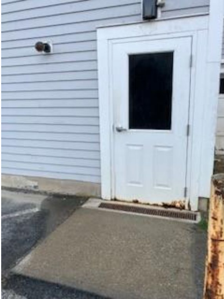
The rear exterior entrance to Tyringham Town Hall. There is a cement landing in front of the door. The threshold to enter the door is over 1 inch above the ground.
