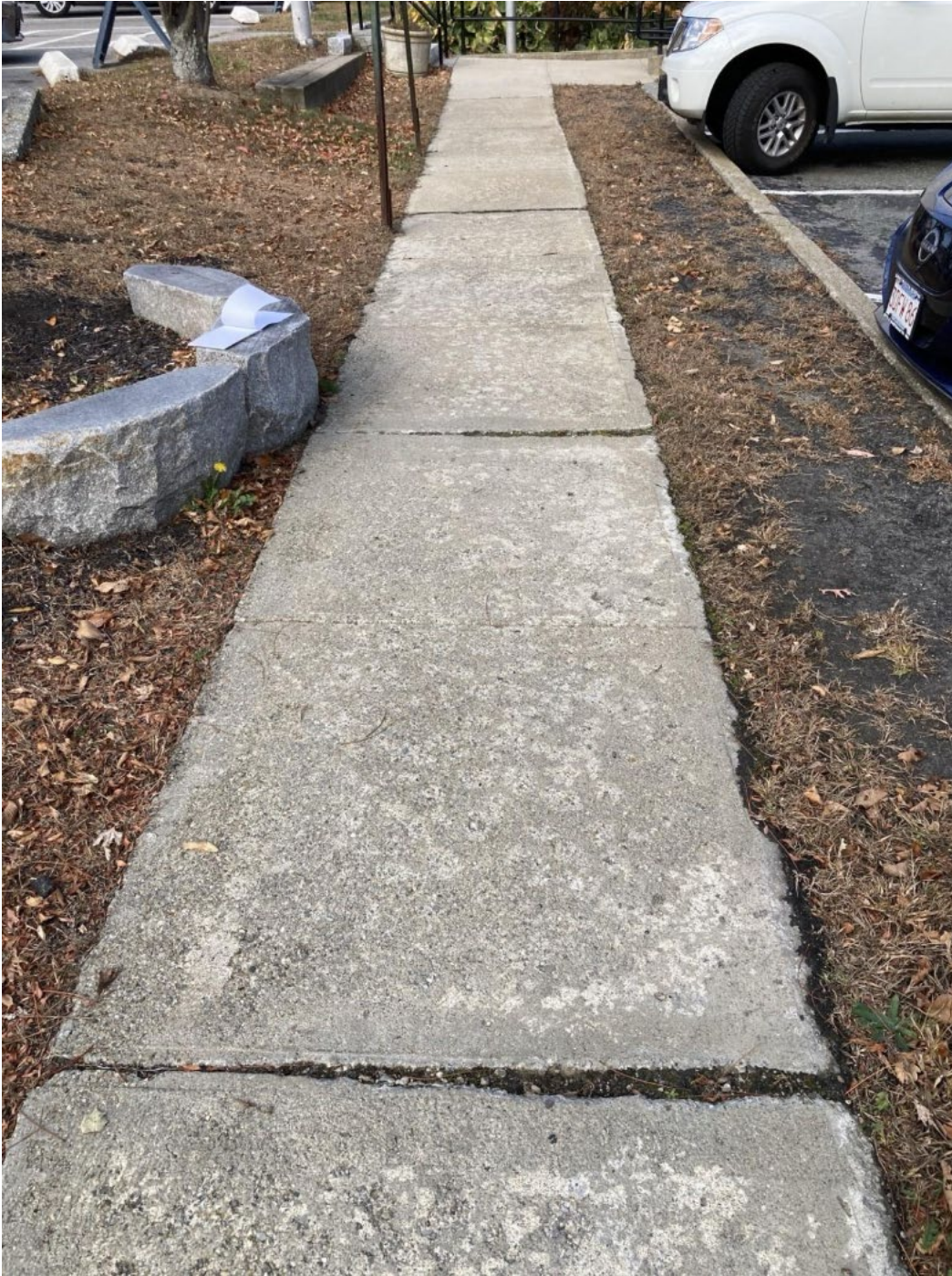
The uneven sidewalk leading to the Rockport Town Hall Annex.
