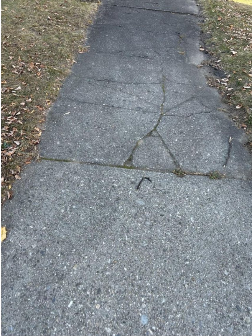
The sidewalk in the path of travel to Saint Paul's Parish. The pavement is cracked and caved in.
