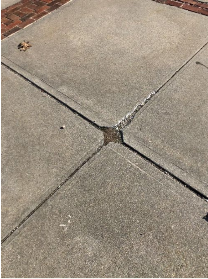
The path of travel to the Corpus Christi Parish Hall. The area where four slabs of cement meet has a crack interrupting the path of travel.
