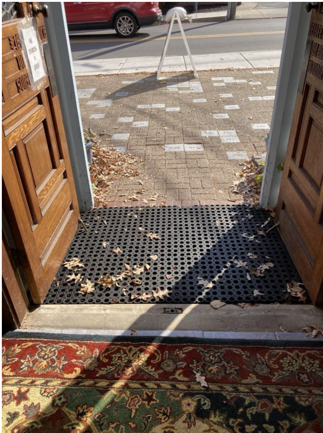
View of the entryway of Saint Mary's Church from the inside of the building, facing towards the street and brick area in front of the church. A concrete threshold of roughly ½ inch to one inch tall disrupts the path of travel.
